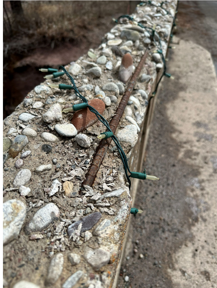
Existing delaminated bridge rail showing rounded river rock aggregate and corroded exposed rebar
