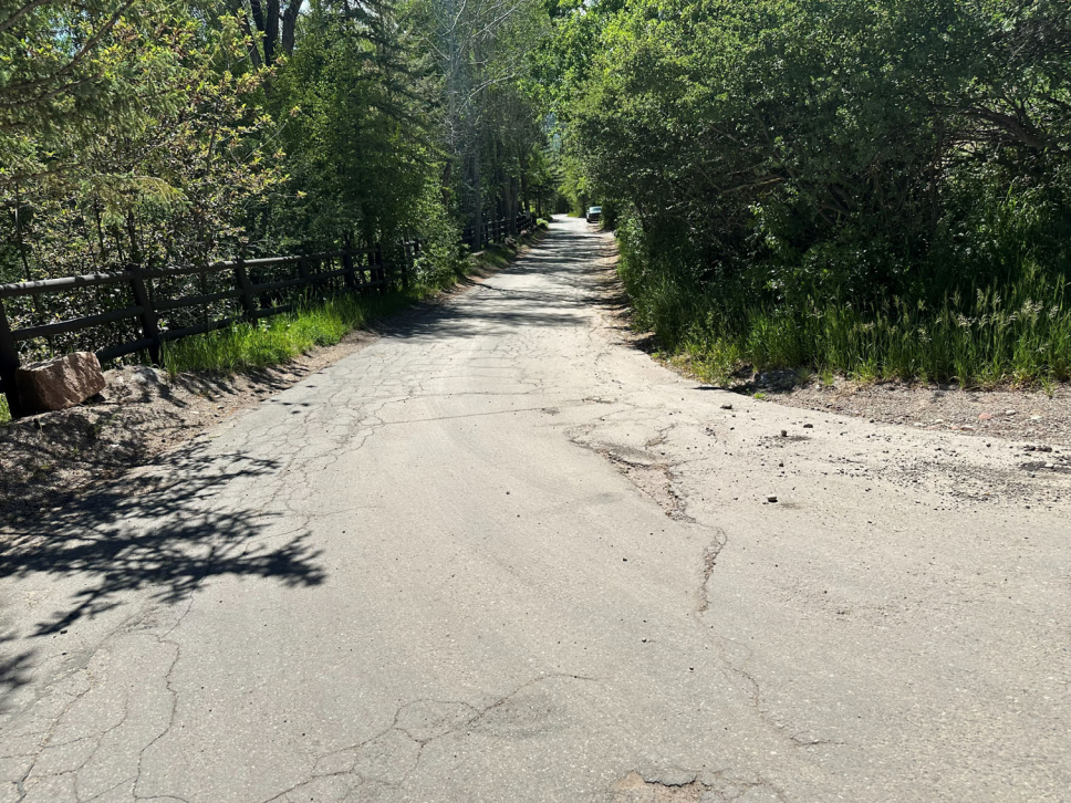
Top section of pavement on Red Mountain Rd, completely failed asphalt and inadequate drainage
