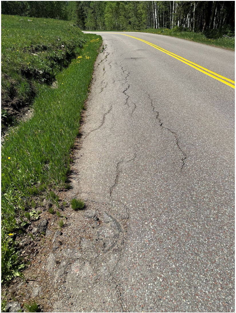
Section of Castle Creek Rd failing due to persistent moisture and poor subgrade
