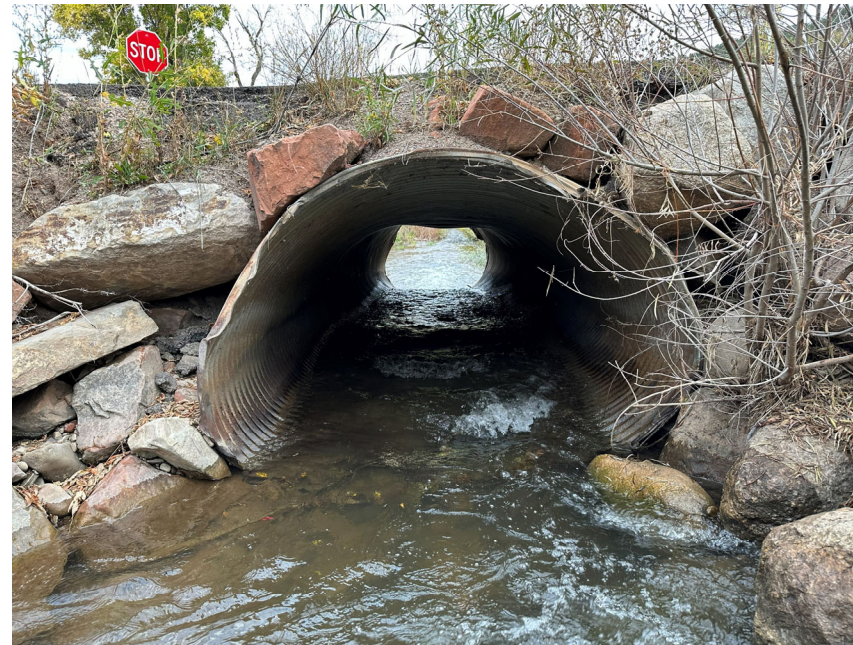
Existing culvert with damage to crown, flowline, and inlet
